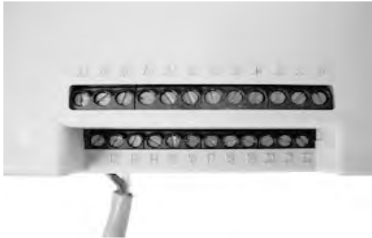
Figure 3.10 PF Softstarter Control Terminals
